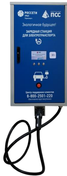
MOUNTED FAST CHARGING STATION
